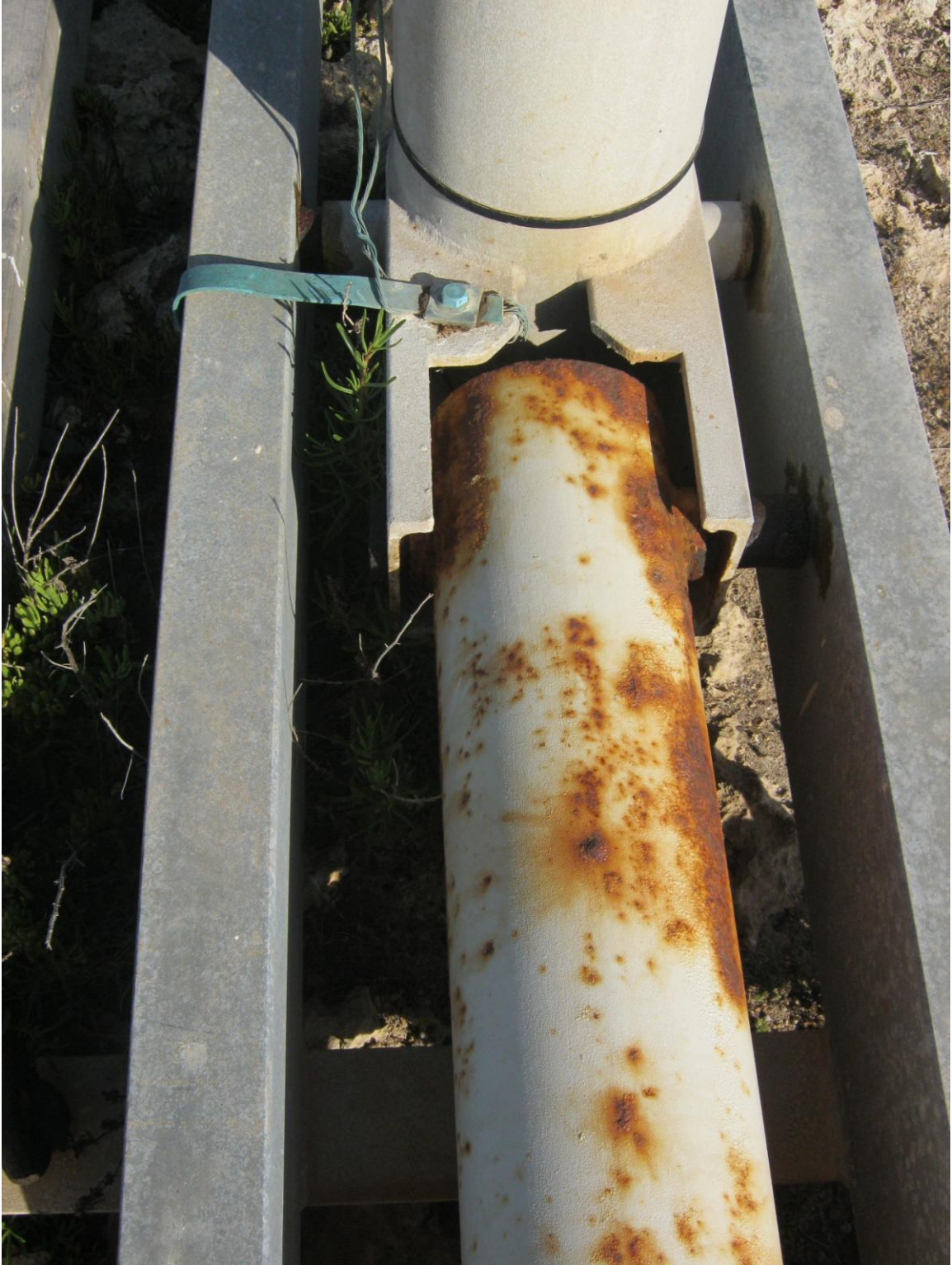
Figure 2- Older gin-pole assembled to main mast once erected. This gin-pole had been replaced in June 2012
