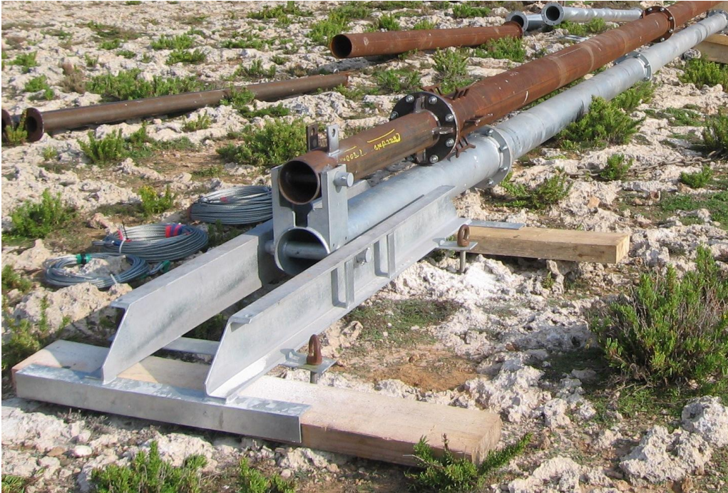
Figure 1 - Older gin-pole assembled to main mast. This gin-pole had been replaced by a new galvanized version in June 2012
