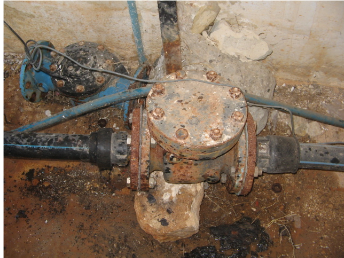
Figure 2. Rusty flange at the Wied il-Qlejjgħa Pumping Station
