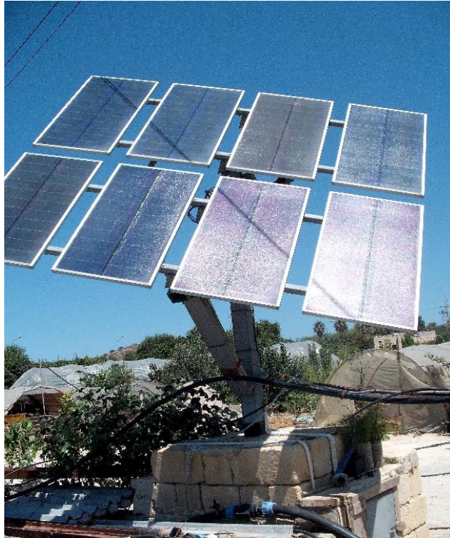
Figure 4. Solar power operated water pump in Mosta
