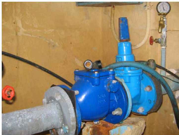
Figure 3. Clean and well maintained pipe system components at Sajjem (Gozo) Pumping Station
